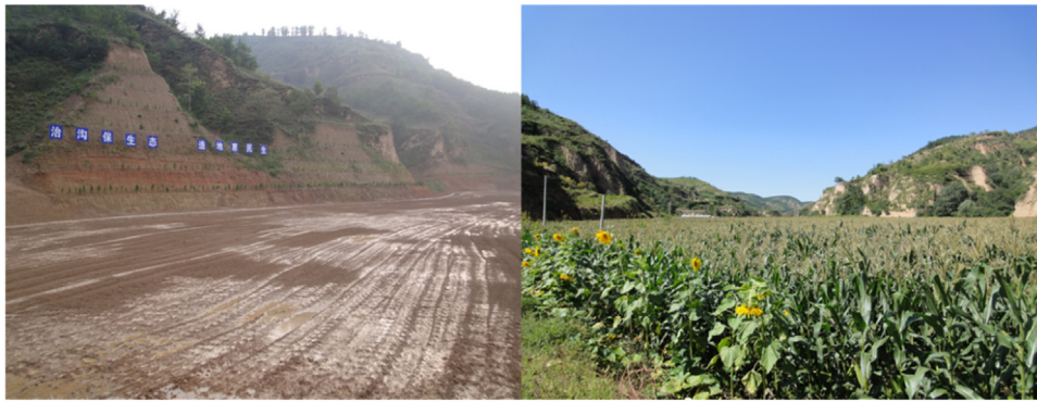
Fig. 6. A gully reclamation project under construction (left) and after the planting of crops (right) (photos by courtesy of Yurui Li, CAS).
